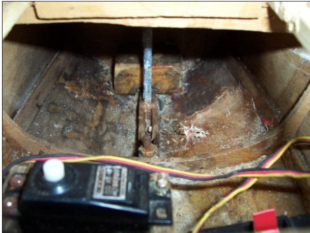
The keel was retained by a 3/16 inch steel rod. A crack all round the hull/keel joint suggested this was not a very stiff mounting arrangement.
