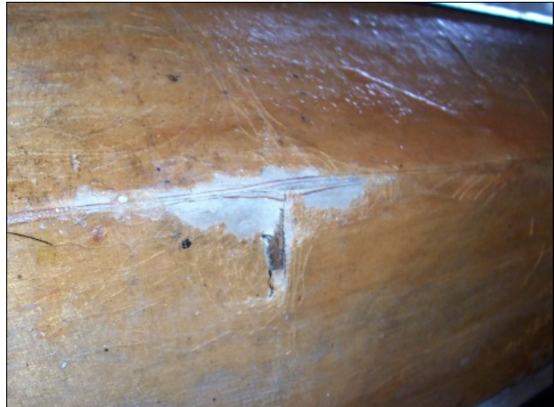
One of three holes in the bottom of the hull. These were patched on the inside with thin plywood before the hull was lined with fibreglass mat, tissue and resin.
