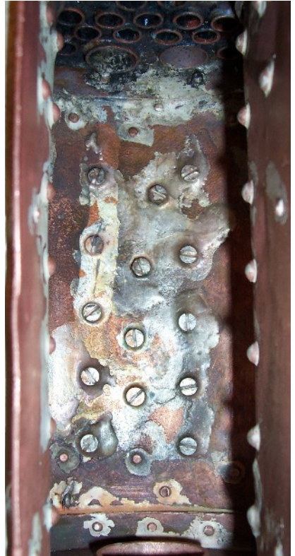
The view inside the firebox. The ten new rod stays are easily visible with the four 4BA screws down the middle (not in a straight line to hit the centre Tee girder stay flanges).
