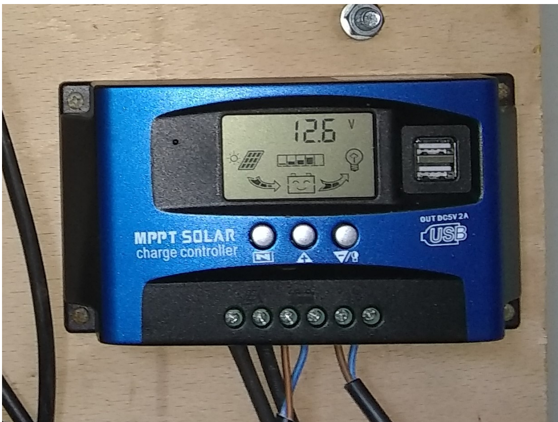
This is the solar charge controller. The LCD display is showing the battery voltage at 12.6V, 80% charged, solar panel is charging, and the load (the LED lights) is drawing power.
