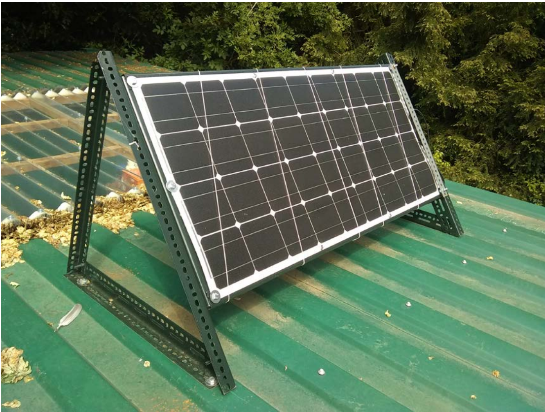
The 32 cell solar panel on the roof of container No 1.
